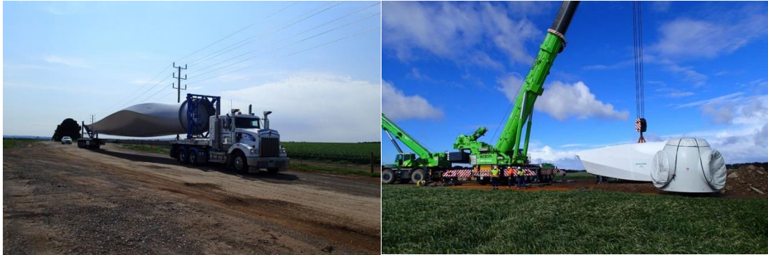
LEFT: a blade delivery; RIGHT: the 500 ton crane unloads and positions the hub and nacelle.
